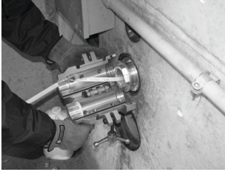
Figure 9 Install Winchline Blower Body
